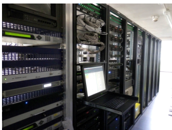
(The server room)
